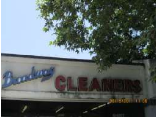
Before: Dilapidated façade.
