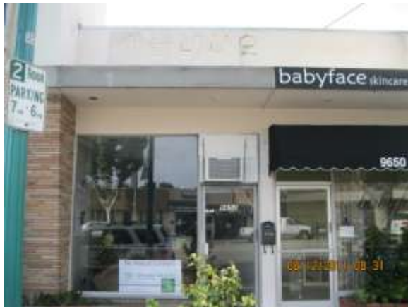
(Before) Sign residue from prior business (front façade).
