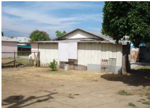
Unpermitted garage room addition. (Before)
