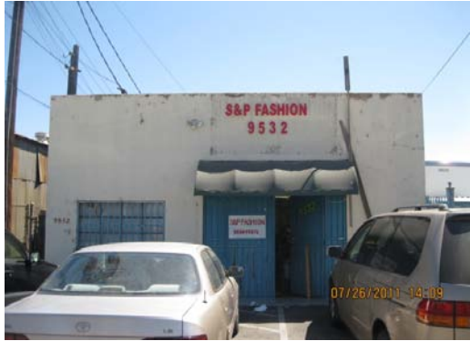
Chipping and peeling paint. (Before)
